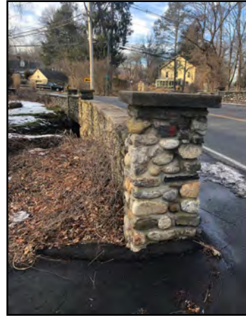
Figure 6: Greens Farms Road Bridge – View of Post at East Side Looking NW
