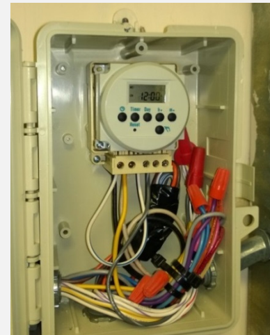
Energy Management System Improvements
