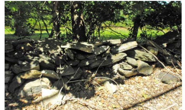
Figure 3-7 A section of existing stone wall requiring repair.
