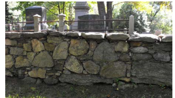
Fig. 3-8 The Lower Green’s Farms Colonial Burying Ground provides an example of stone wall restoration.
