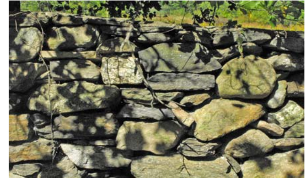
Figure 3-6 A section of existing stone wall along Green’s Farms Road in good condition.
