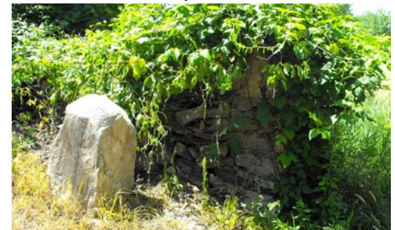
Fig. 3-13 Invasive vines should be removed from the stone walls.
