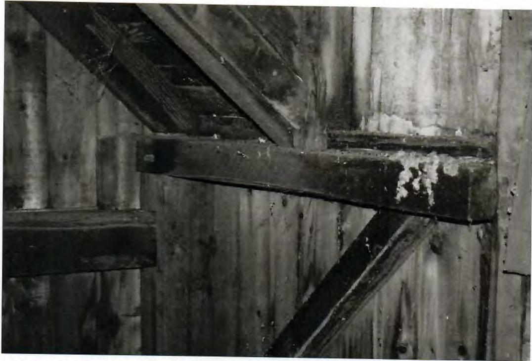
15. Detail of the interior, northwest corner, showing dropped tie-girt in end wall. Note how the rafter plate is truncated for the shed dormer.
