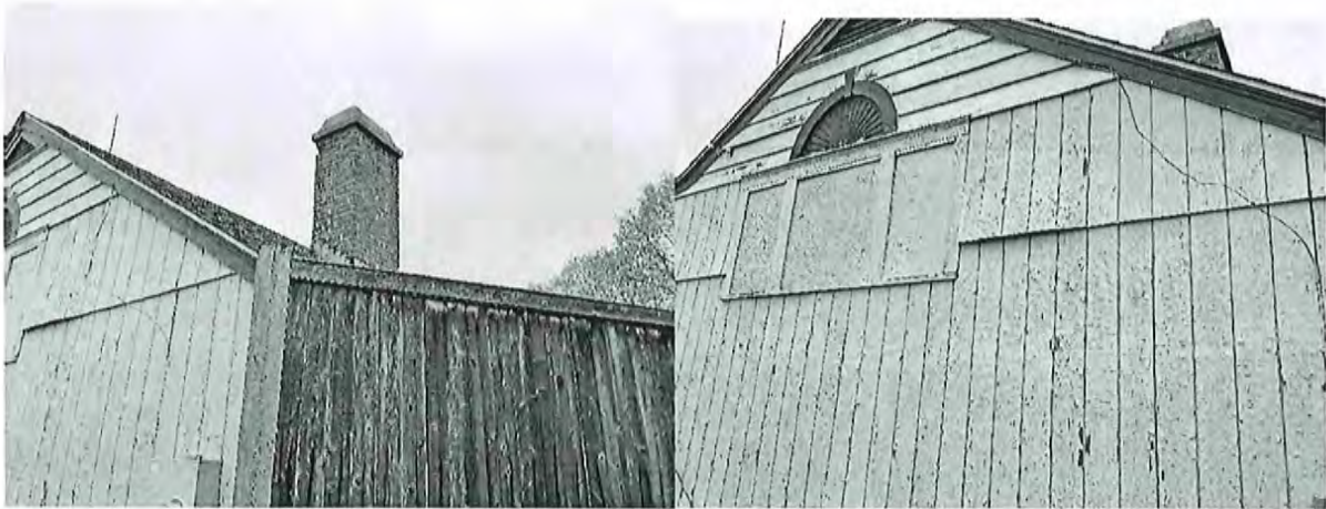
Chimney needs repointing.
