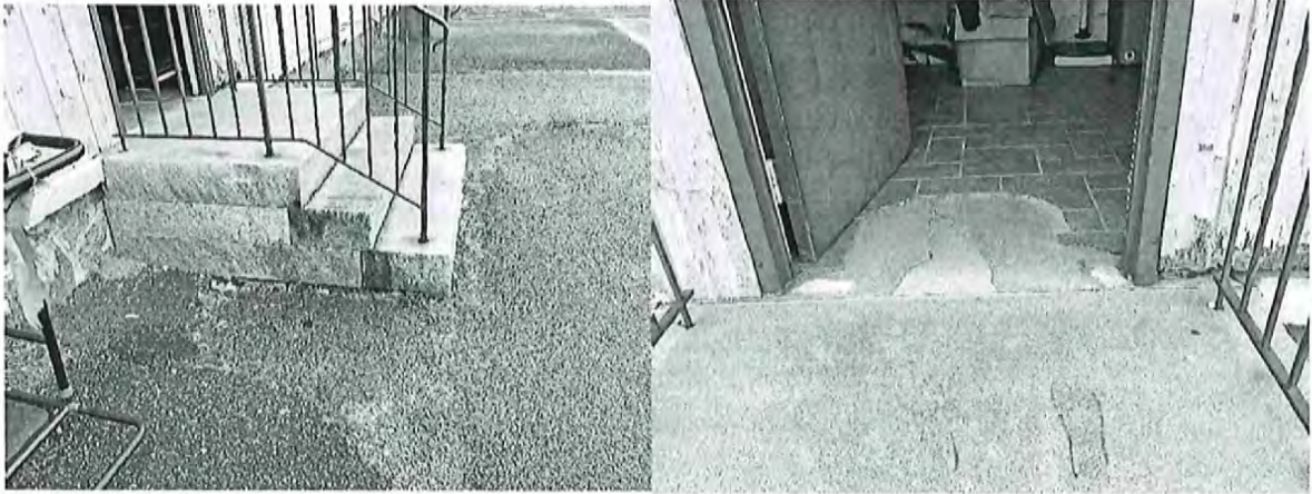
Front steps and walkway are adequate. Damaged floor tile at entryway.
