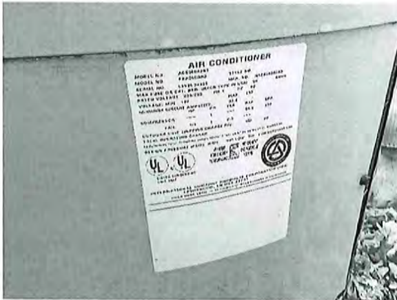
AC condenser unit not tested.
