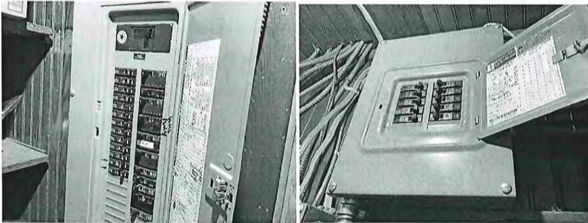
200amp electrical panel and sub panel.
