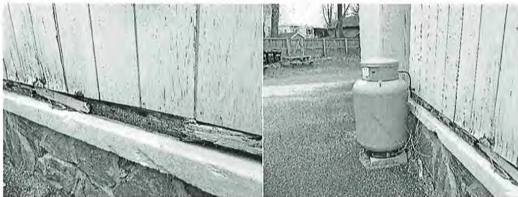
Rotted sill plate needs replacing. Propane tank for Concession appliances appears okay.
