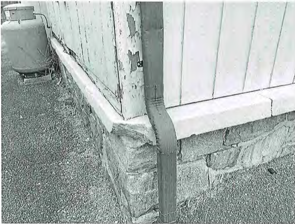
Cap stone on foundation is damaged also the foundation needs to be repointed.
