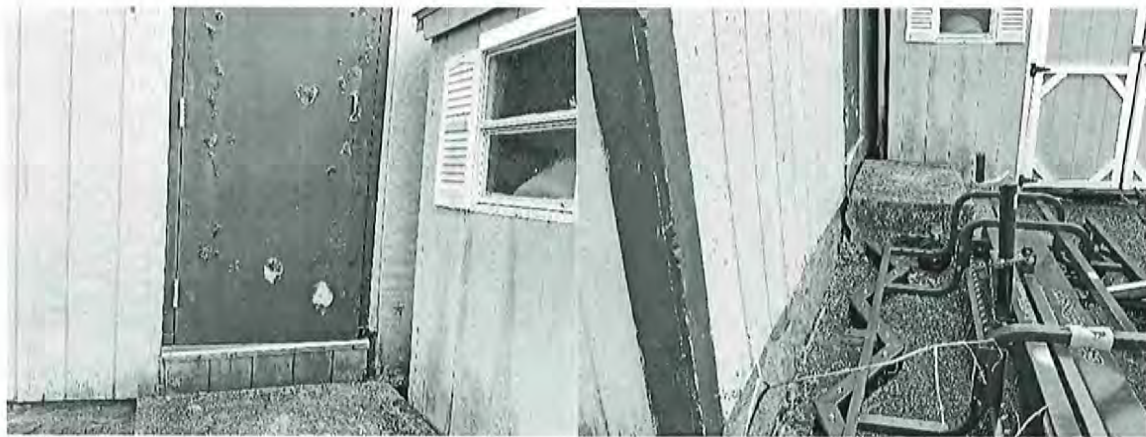
Rear exterior door should be repaired or replaced. Rear steps are pulling away from the building.
