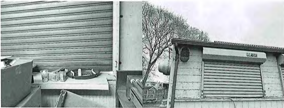
Concession rollup doors; seams are failing.
