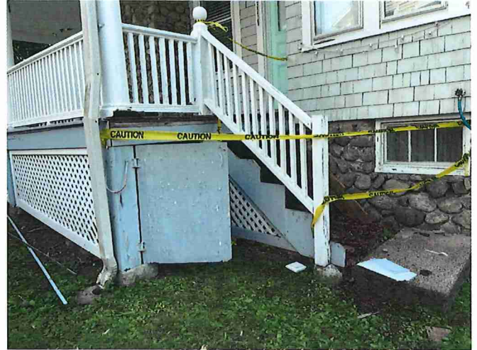
Rear stair has collapsed.
