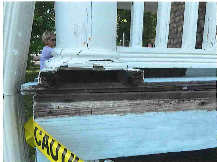
Deterioration of load bearing base of corner post.
