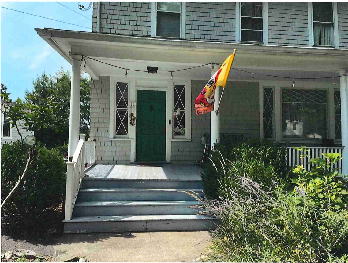
Front steps are collapsing on the right side & require foundations under the existing circular columns.
