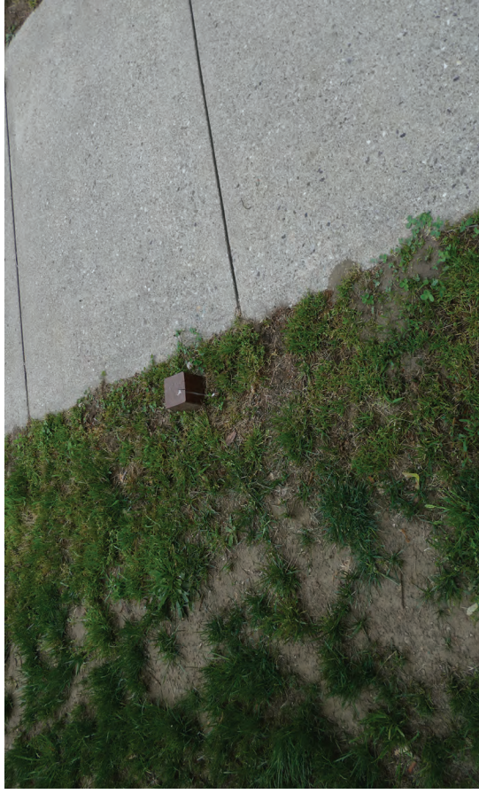
POTENTIAL TRIPPING HAZARD.
