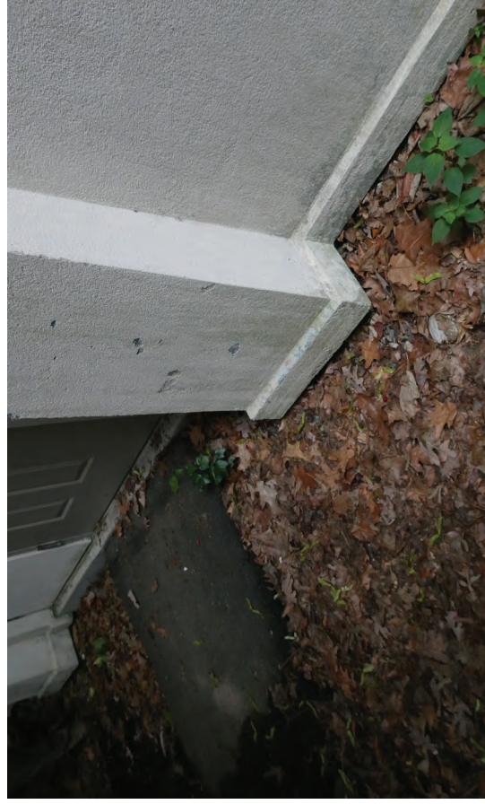
SOME EFIS PATCHING AND PAINTING NEEDED.
