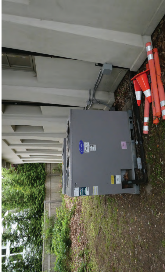
NEW CONDENSOR UNITS
