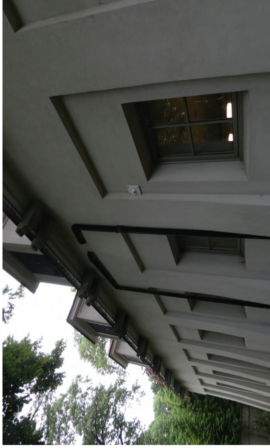
DRIP GUARD TO BE CLEANED.
