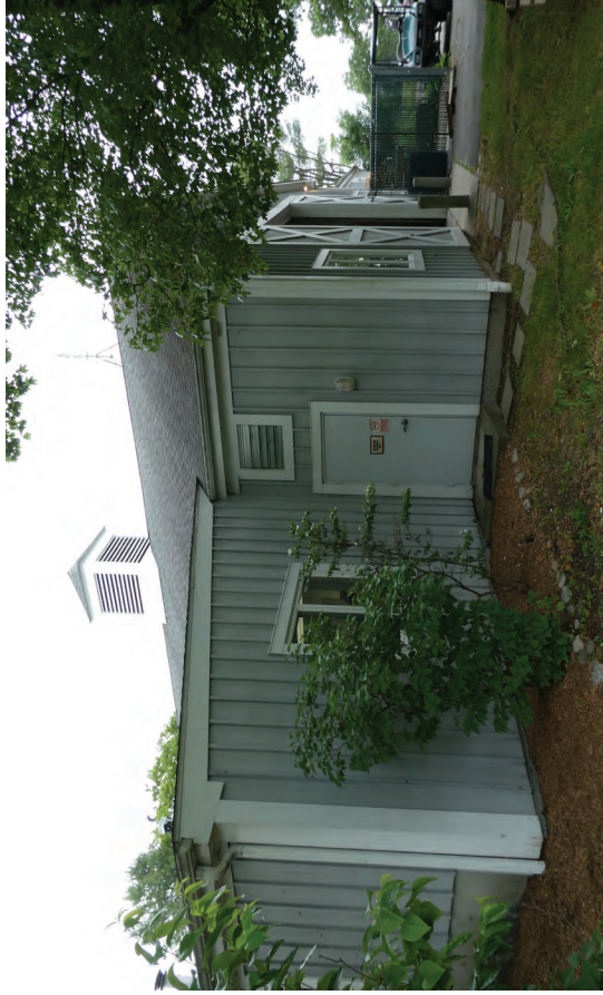
EXTERIOR WALL REQUIRES REPAINTING SOON.
