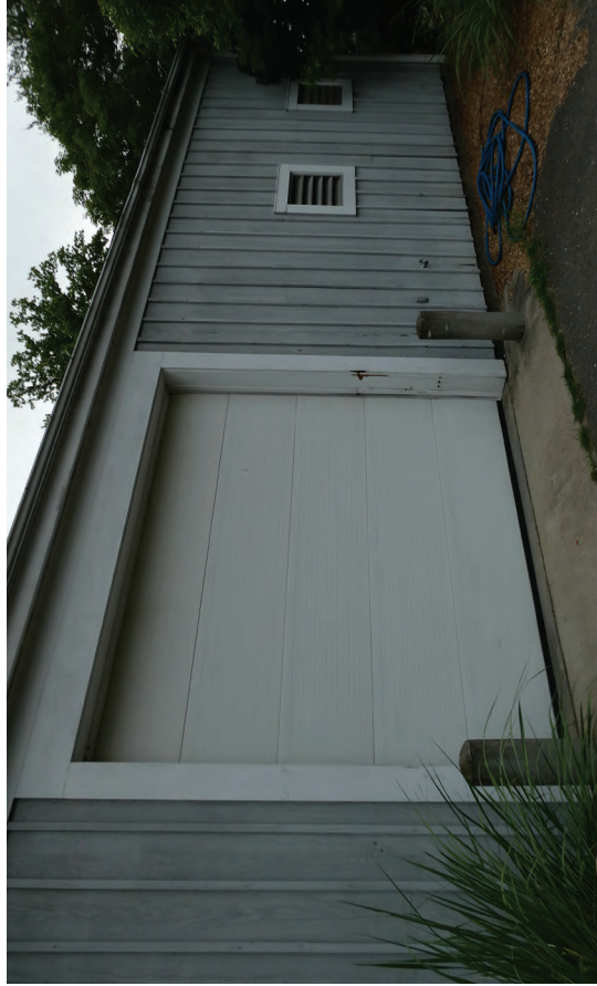
PAINTING OF TRIM AND SIDING REQUIRED.
