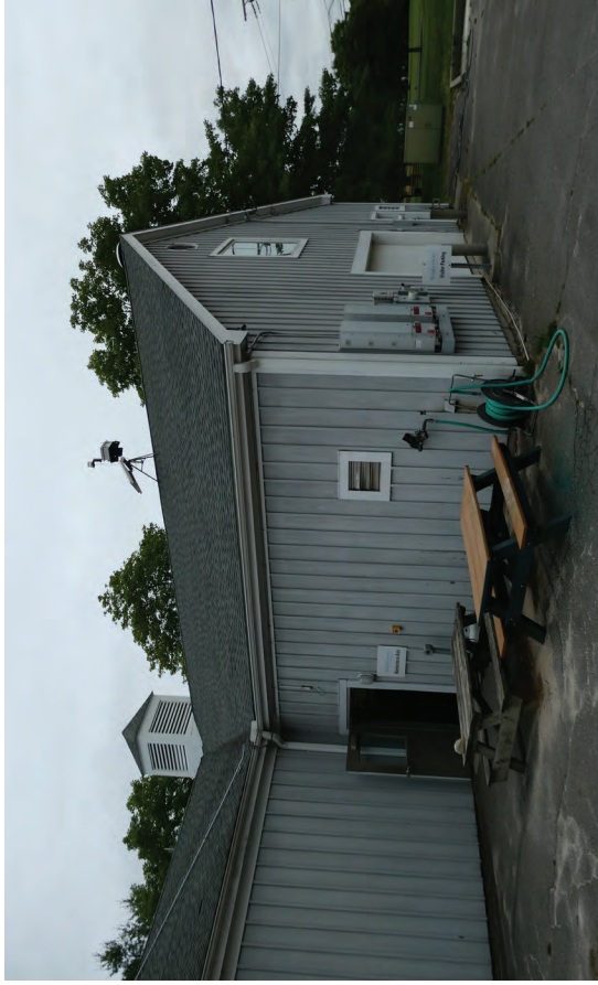
COURSE LIGHTING PROTECTION SYSTEM IN TACT.
