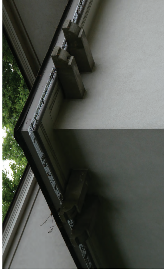
BEAM ENDS TO BE PREPARED AND PAINTED.
