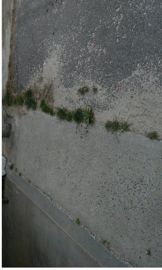
SOME PAVEMENT IMPROVEMENTS NEEDS.
