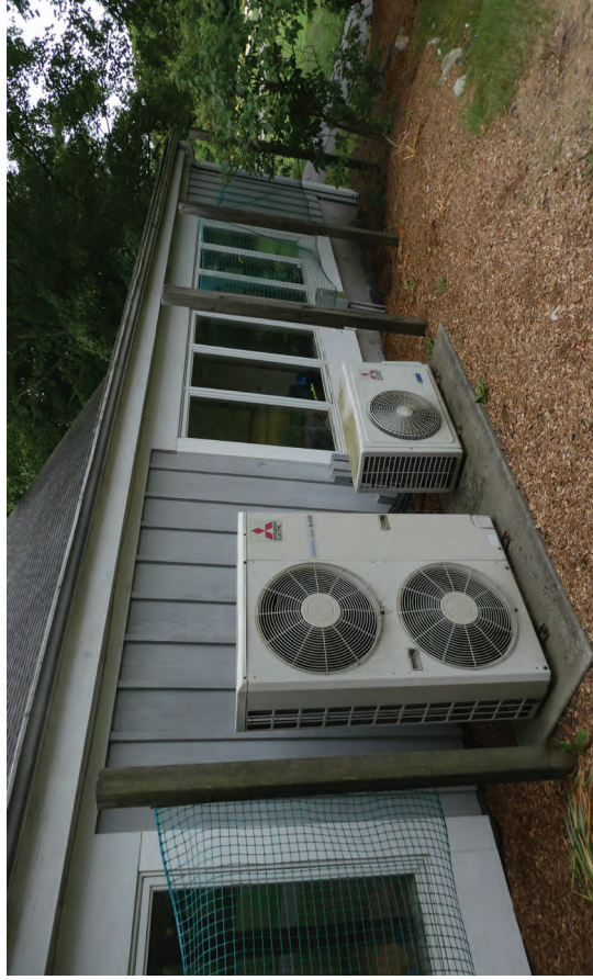
CONDENSORS ON WEST SIDE.
