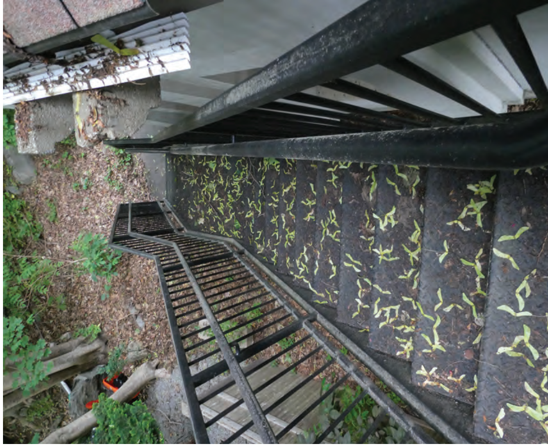
FIRE EXIT STAIR TO BE CLEANED.
