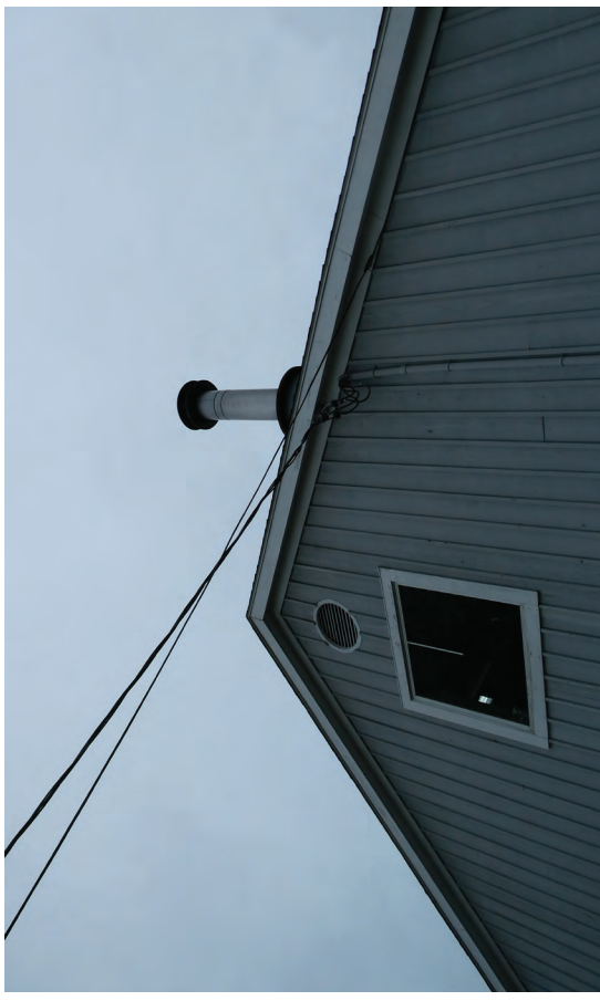
WINDOW TRIM BROKEN.
