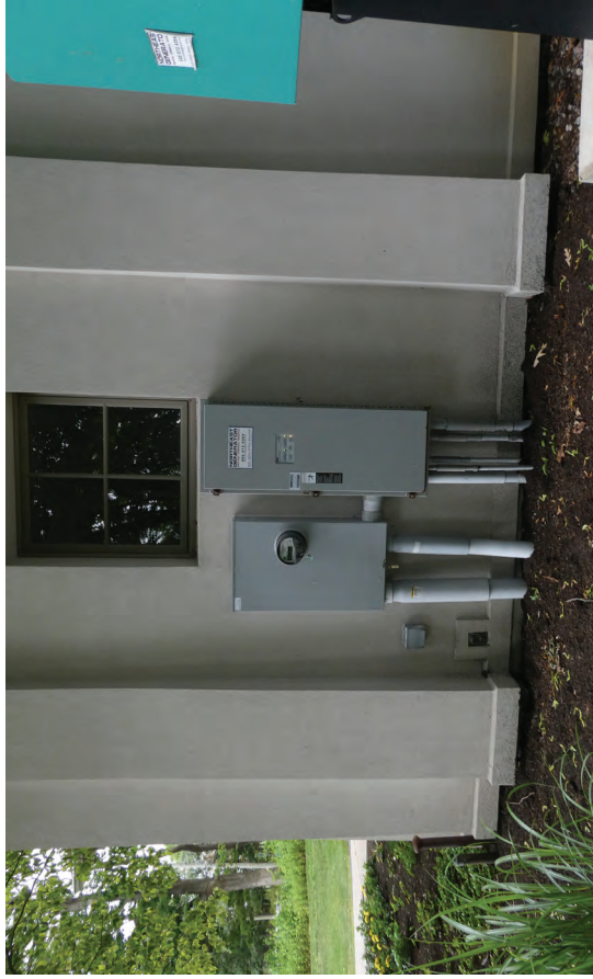
NEW SWITCH GEAR
