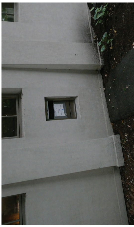
FACADE CLEANING REQUIRED.
