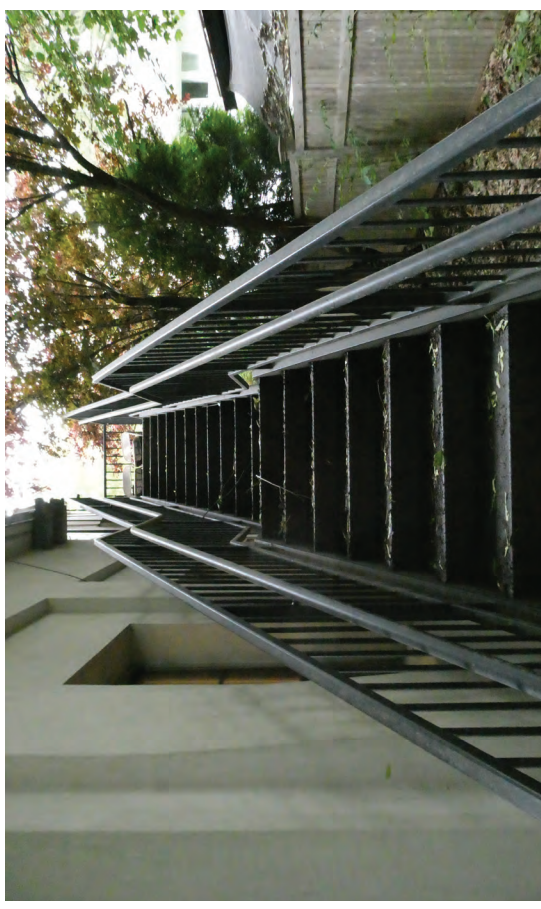
EMERGENCY STAIRS TO BE KEPT CLEAN.
