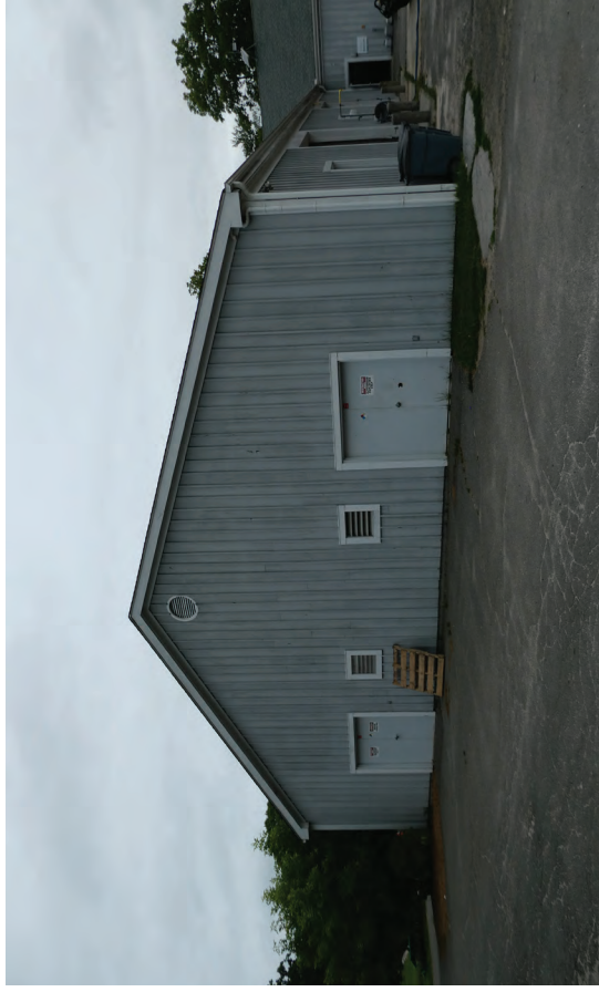
EAST FACED REQUIRES PAINT SHORTLY.
