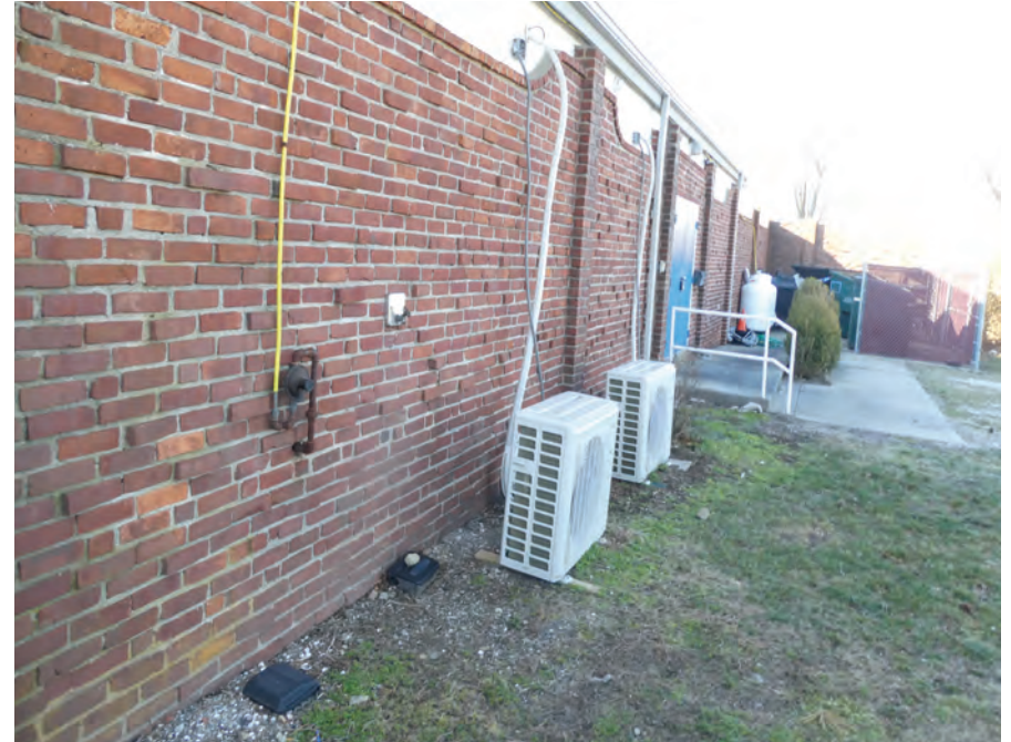
CONDENSOR SHOULD BE SCREENED.
