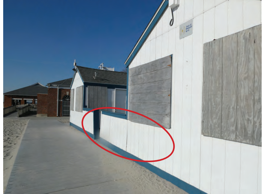
AREA REQUIRED SOME SIDING REPLACEMENT
