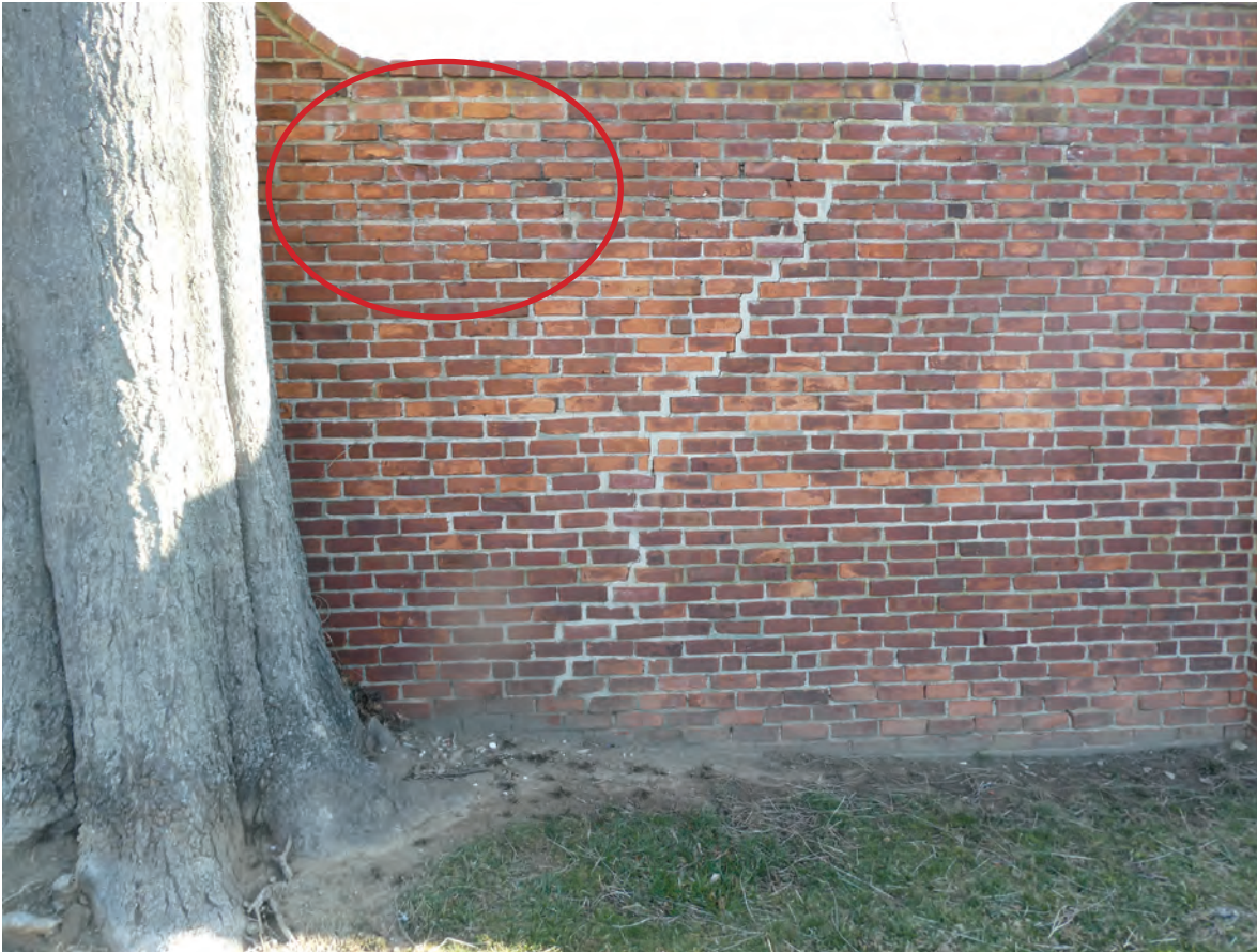
TREE ROOT AFFECTING WALL REPOINTING REQUIRED IN SELECT AREAS.
