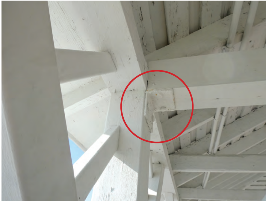
REPLACE RUSTED ANGLES AND TIES
