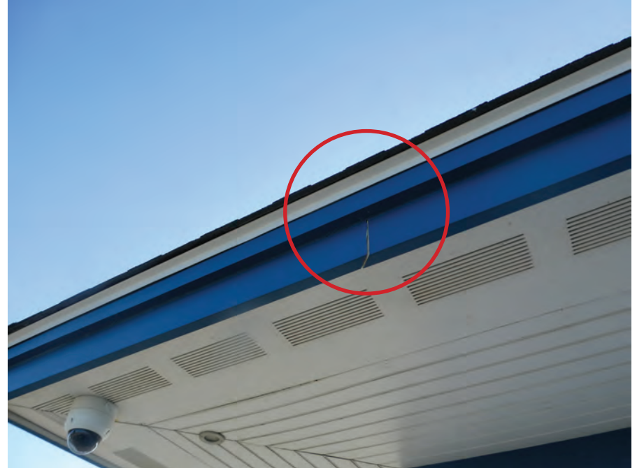
WASH SOFFITS - PATCH BOARD SHRINKAGE.
