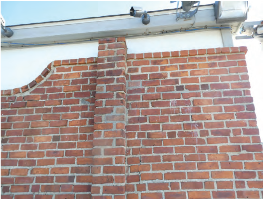
EXTERIOR BRICK WALLS - REQUIRED REPOINTING AND CRACK REPAIR.
