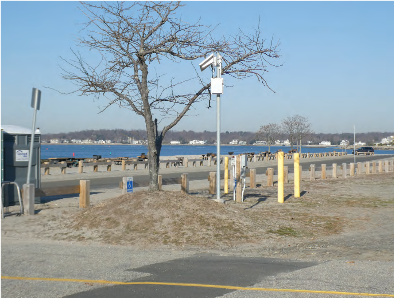
SEWER EJECTOR SYSTEM
