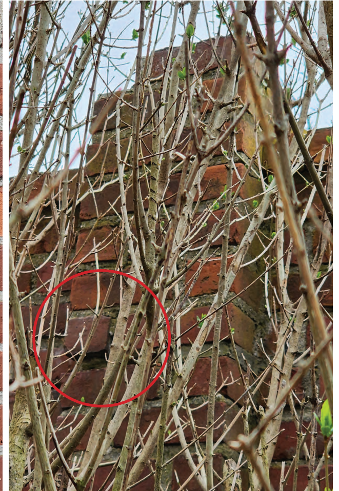
REPOINTING REQUIRED ON WALL.
