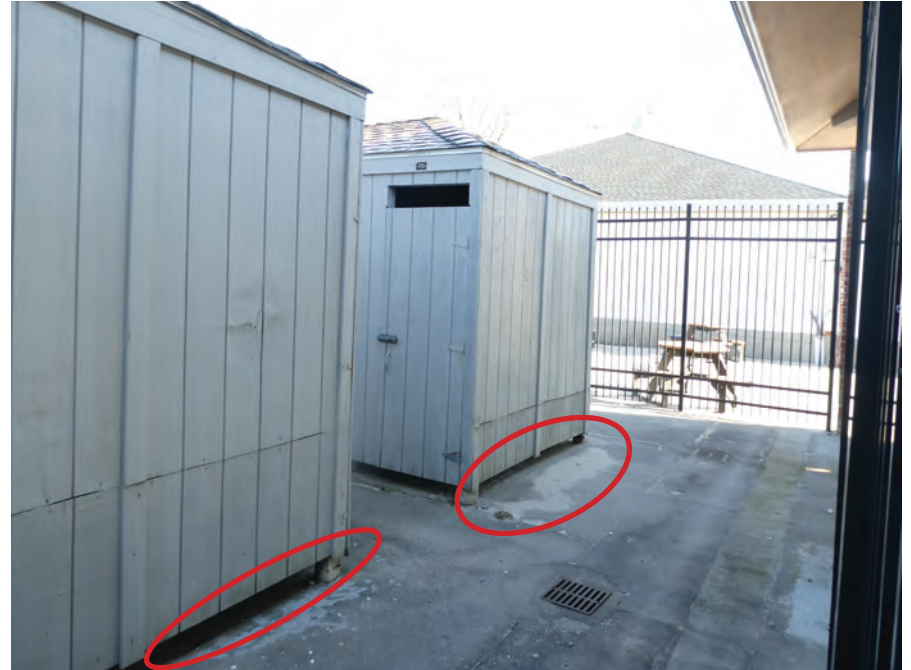
OLD CABANAS FROM WOOD REQUIRED REPLACEMENT - ROTTING IN AREAS
