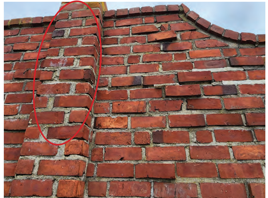
BUTTRESS COLUMN REQUIRED REPOINTING.
