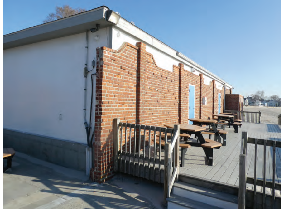
NEWER DECK AREA - SOME TRIPPING HAZARDS.
