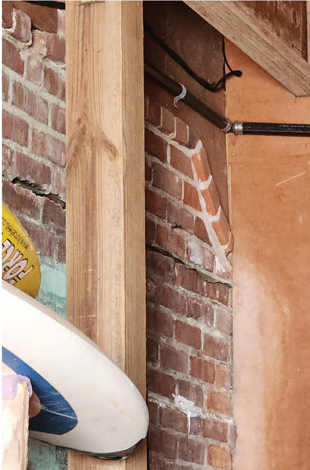
HORIZONTAL CRACK IN WALL.
