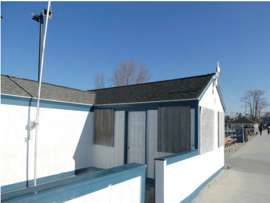
ROOF APPEARS NEWER
