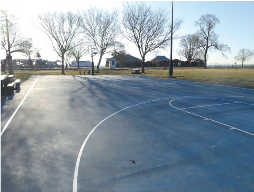
SELECT AREA DETERIORATION
