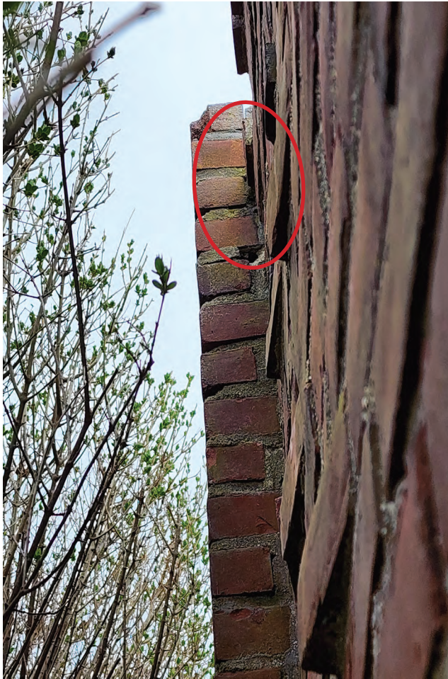
COLUMN BUTTRESS SEPERATION
