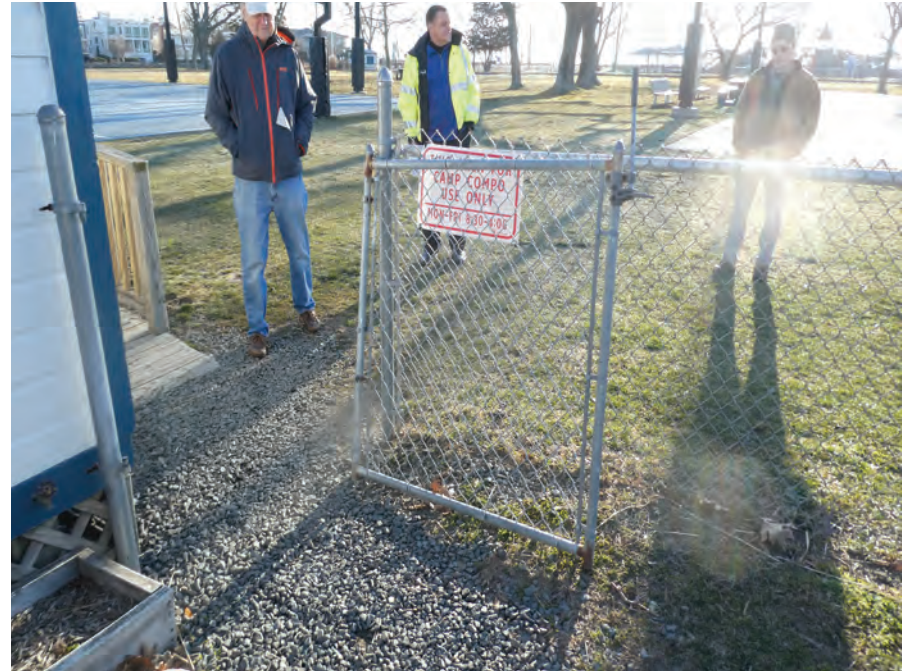
GATE UNHINGED REQUIRED REPLACEMENT.
