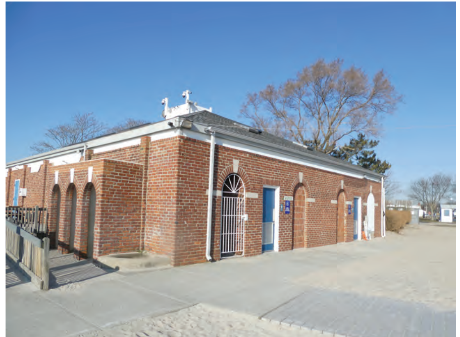
TOILET AREA - REQUIRED REMODELED.
