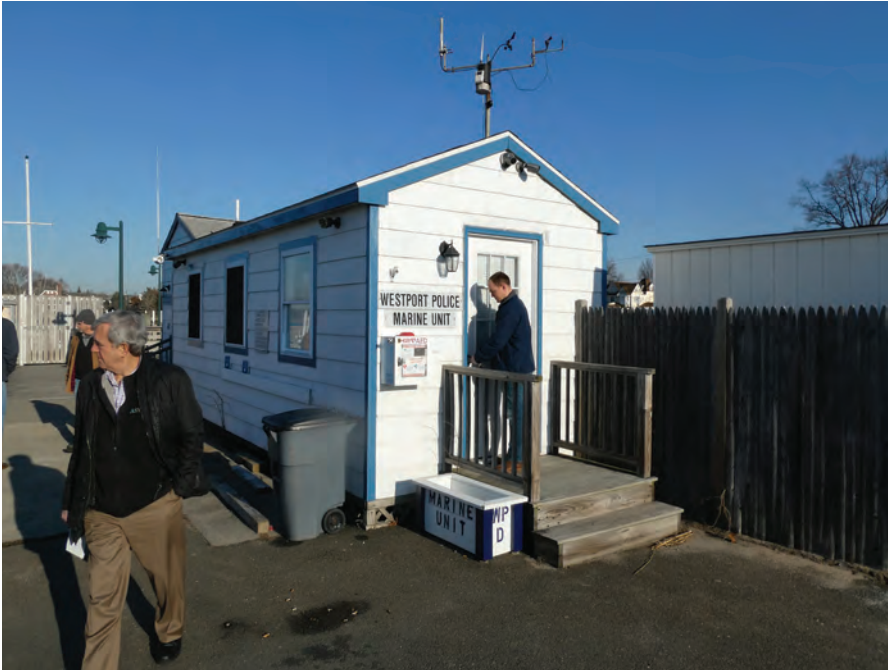
OVERALL BUILDING - EXTERIOR PAINT REQUIRED.
