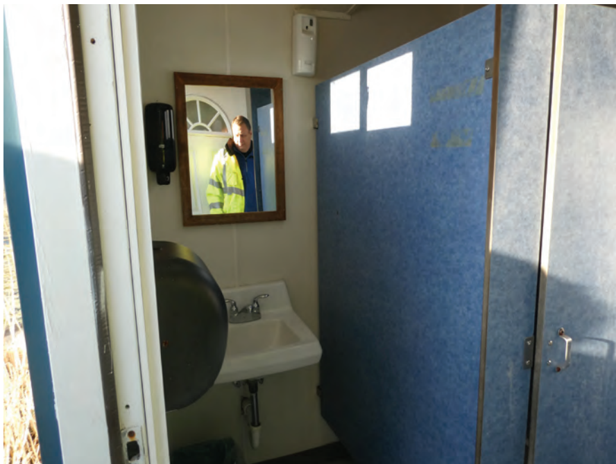
INTERIOR TOILET - SATISFACTORY, NON ADA.
