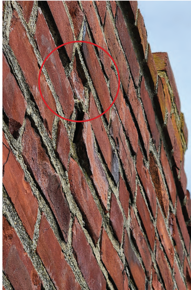
SOME SPALLING BRICK.
