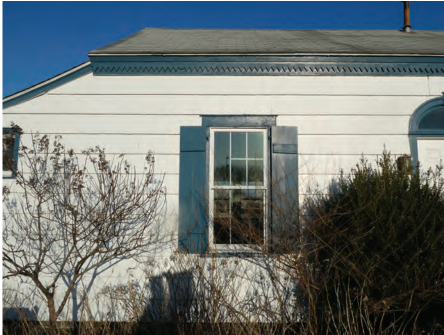
WINDOW MUNTIN BROKEN/OLDER WINDOW.
