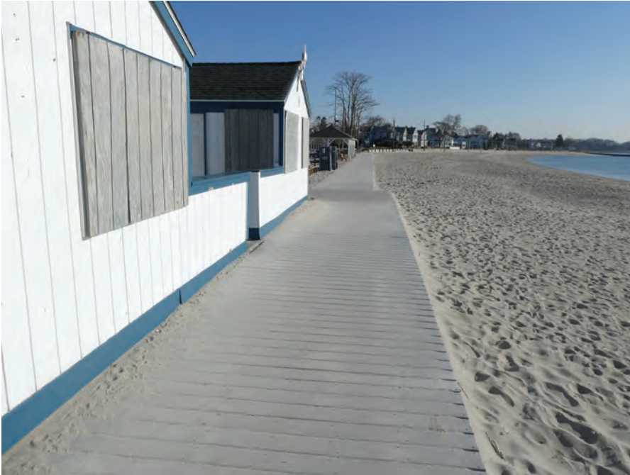
OLD BOARDWALK - REPLACE
