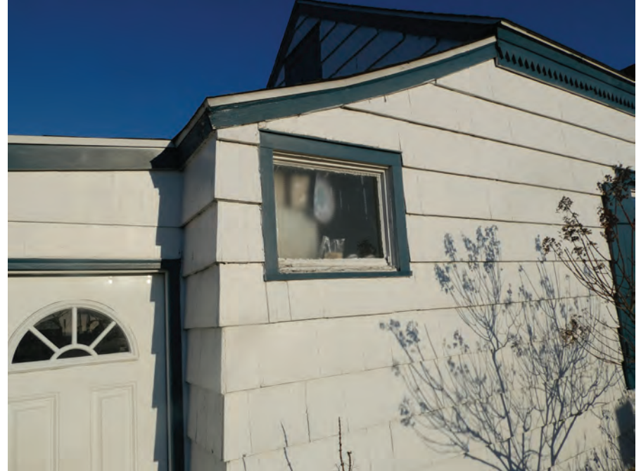
ROTTED SILL AND OLD WINDOW (REPLACE)
