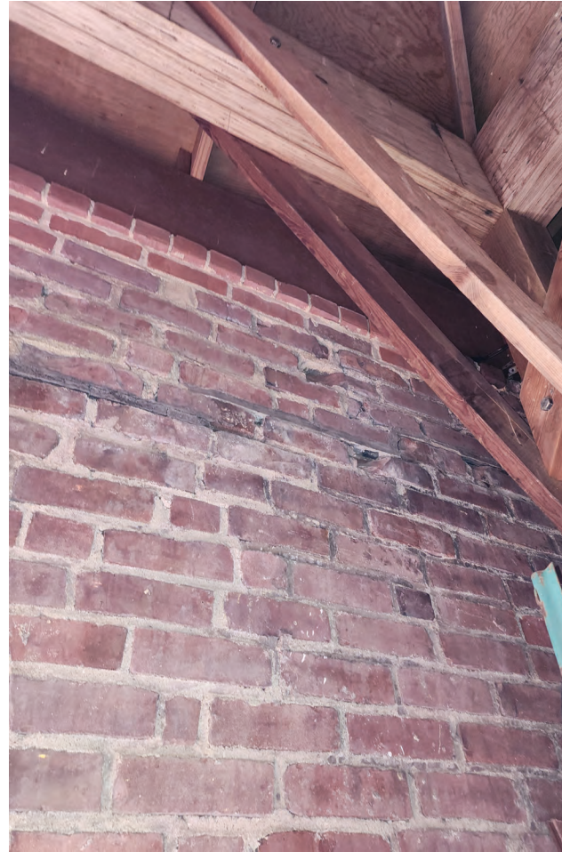
HORIZONTAL CRACK IN WALL.
