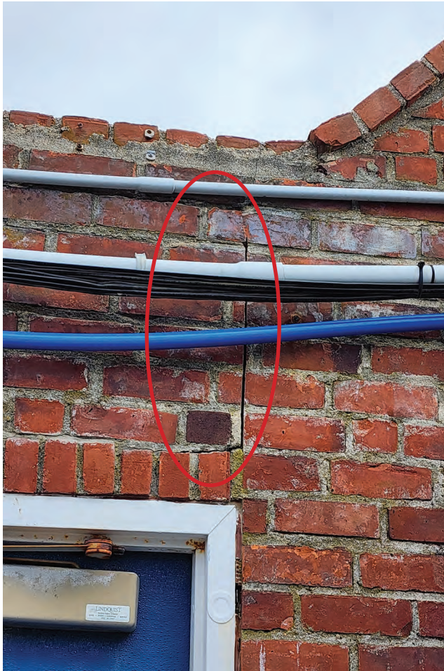
CRACK AT DOOR WALL
