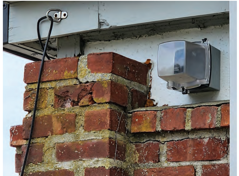
LOOSE BRICK TOP CAP
