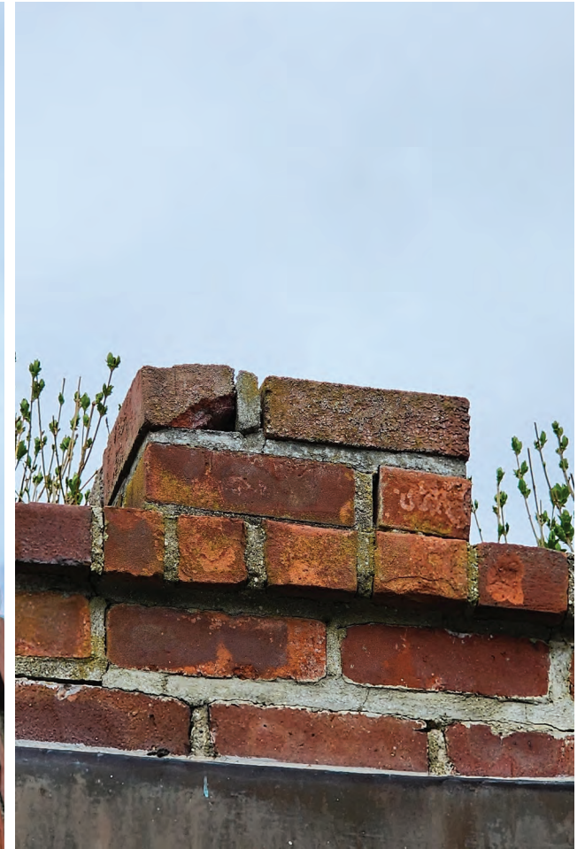
BRICK TOP CAP REQUIRED RESETING (REPAIR)
