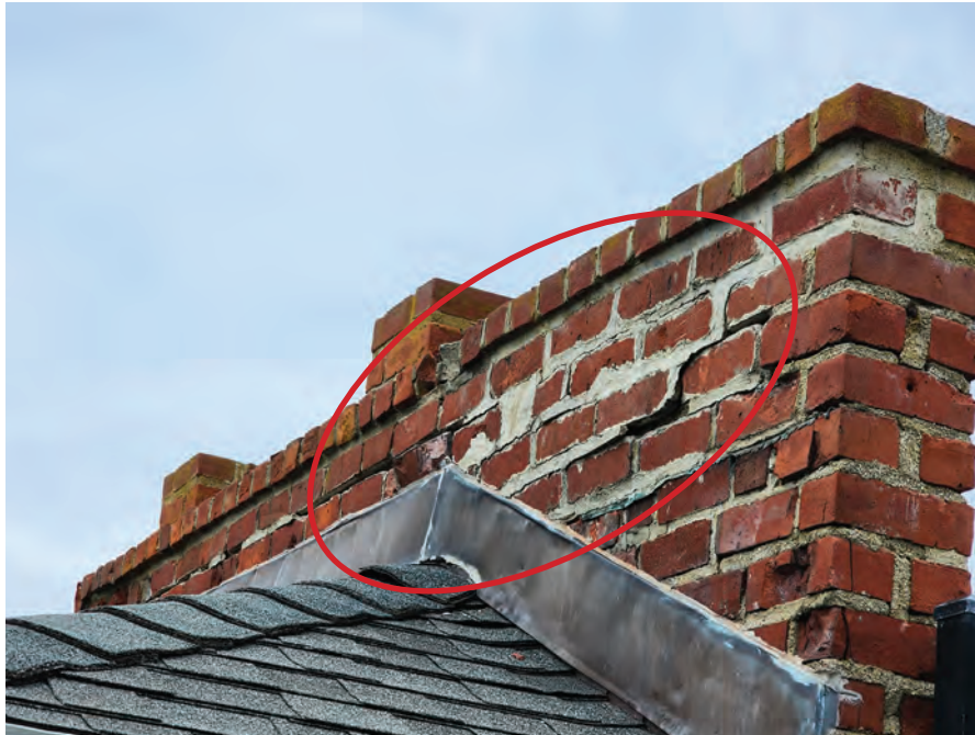
PARAPET REBUILD REQUIRED.
