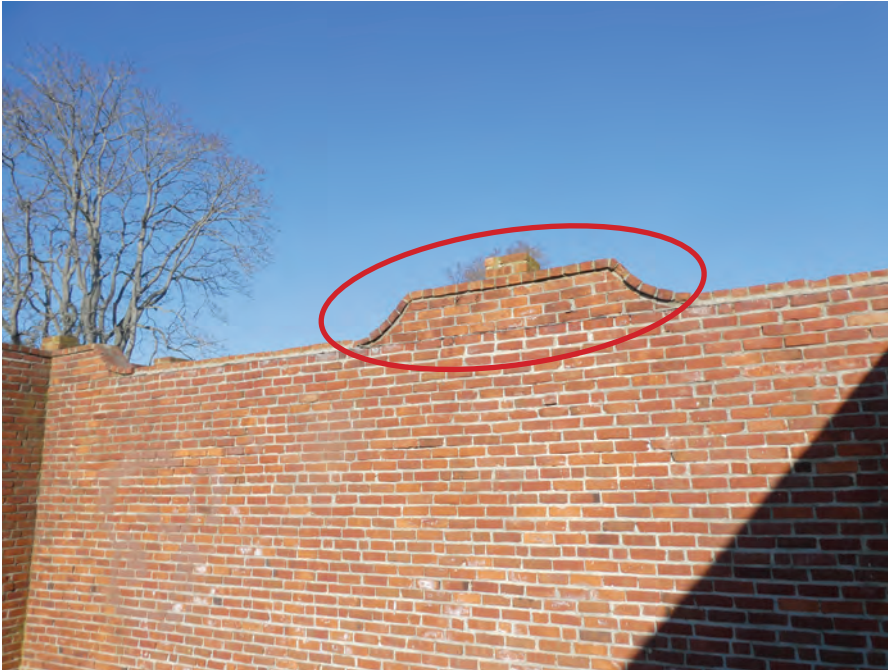
WALLS REQUIRED SOME REPOINTING.
