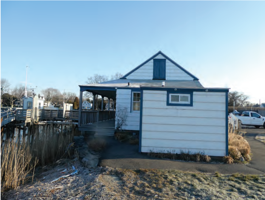
SOME UNEVENNESS IN BITUMINOUS WALKWAY.
