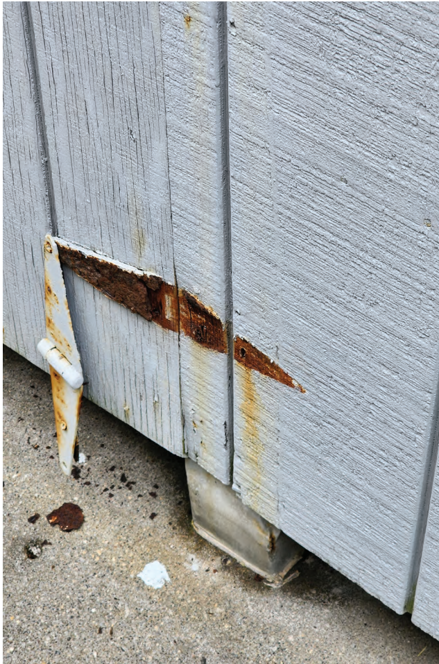
DETERIORATED BATHHOUSE HARDWARE
