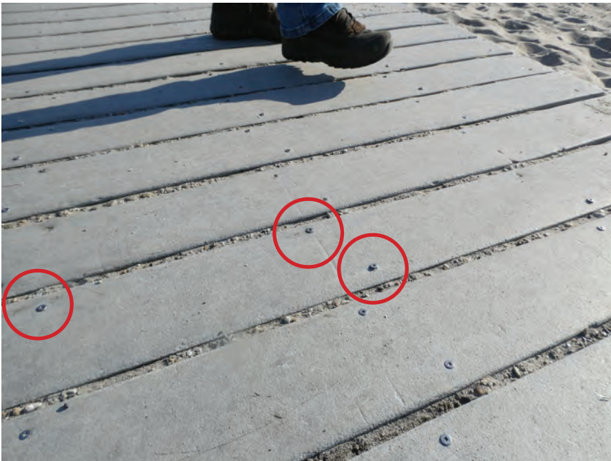
SCREWS PROTRUDING (CANNOT BE ADJUSTED HEADS BREAK)
