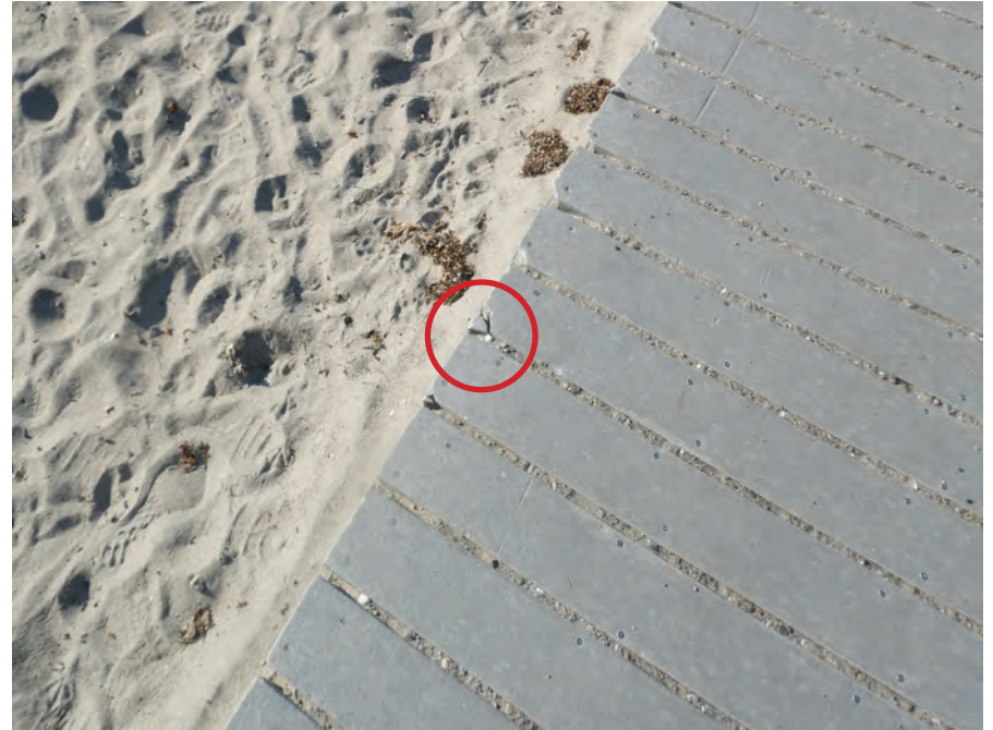
BROKEN EDGES IN AREAS
