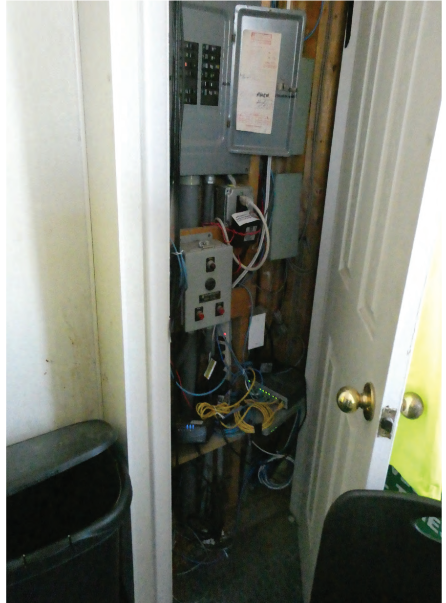
ELECTRICAL SYSTEM REPORTED ADEQUATE.
