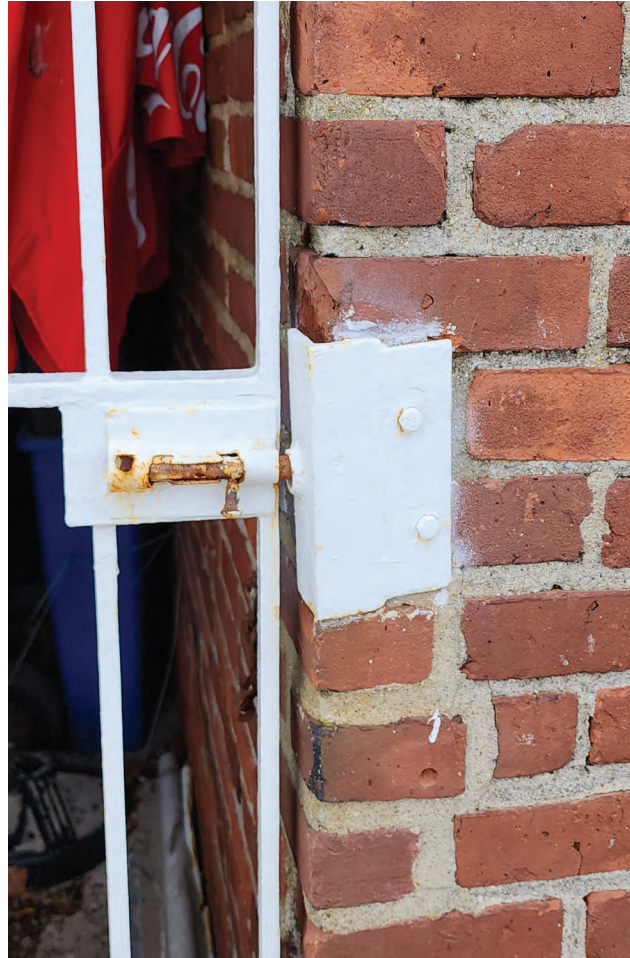
LOOSE GATE LATCH
