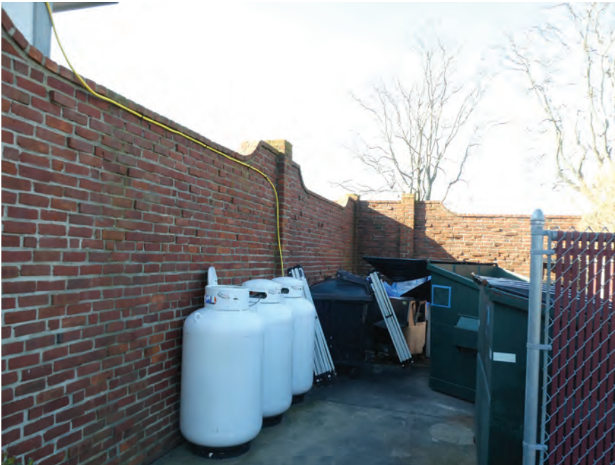
PROPANE TANKS SHOULD BE SCREENED.
