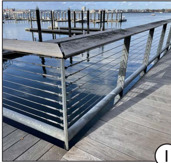
WOOD AND CABLE
