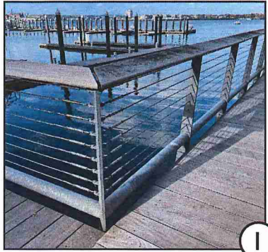
WOOD AND CABLE
