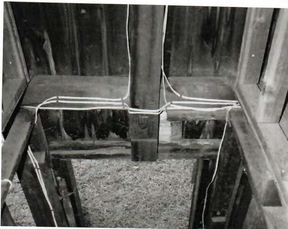
16. Detail of interior, severed post where center entry on south eave-side now is, camera facing south.
