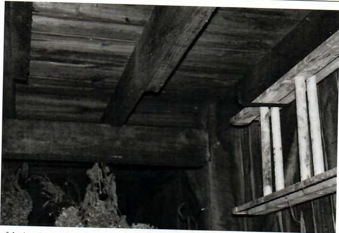
13. Detail of the interior, north wall, main level, square rule construction and circular sawn posts, camera facing east.
