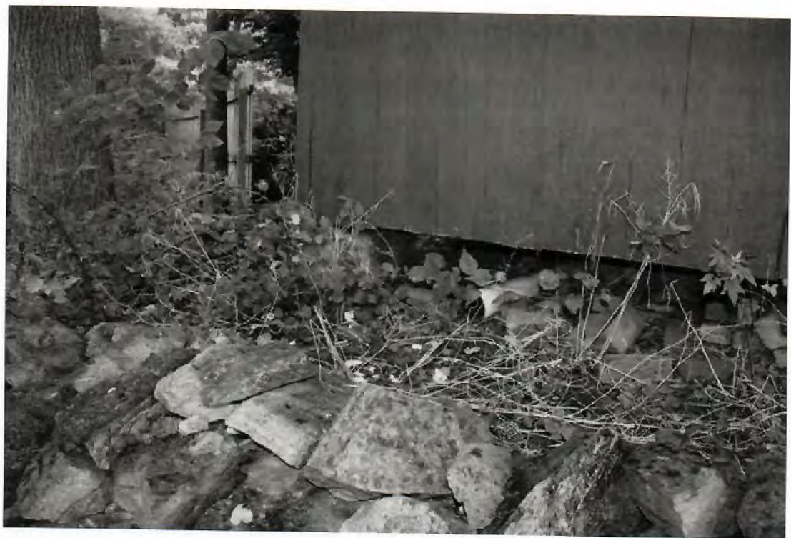
12. Detail of the exterior, northwest corner of the barn. Note the single stone pier at the corner.
