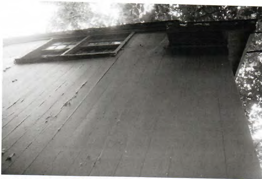
10. Detail of the exterior, north eave-side wall dormer, east corner, camera facing south.
