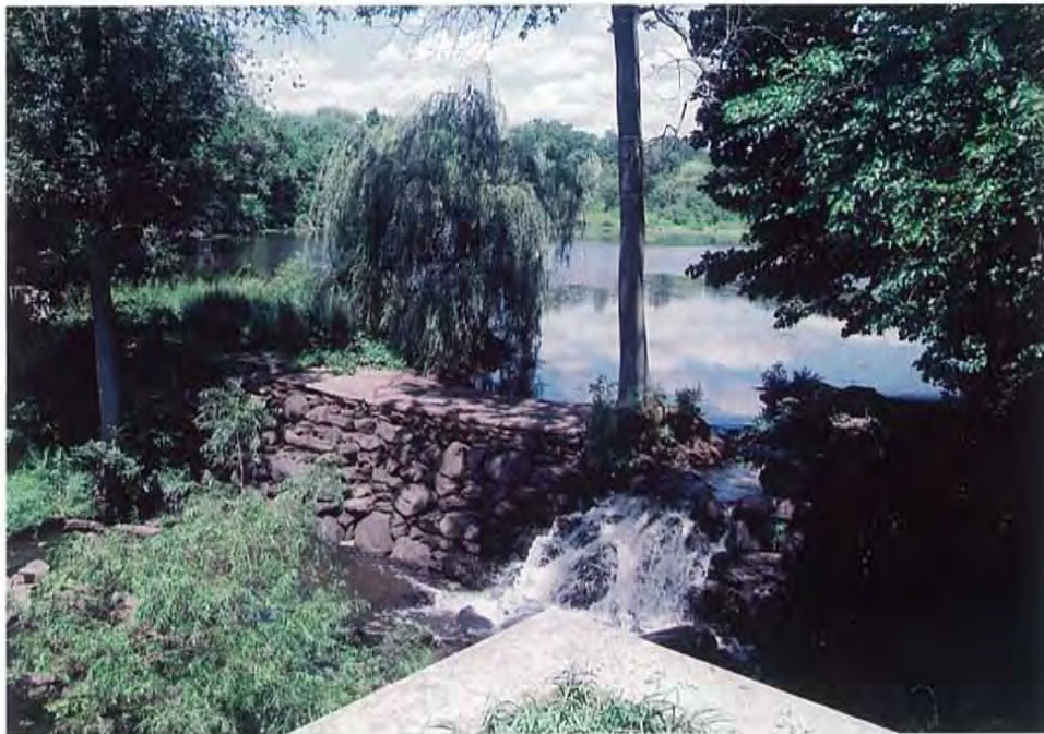
Photo 1-7: The Bulkley Pond Dam formed Bulkley Pond and marks the upstream extent of tidewater in Sasco Brook.
