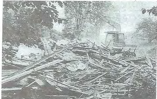
MONDAY, JULY 19: All that remains after a demolition crew leveled the historical landmark. Photos by Curtis Zorn
