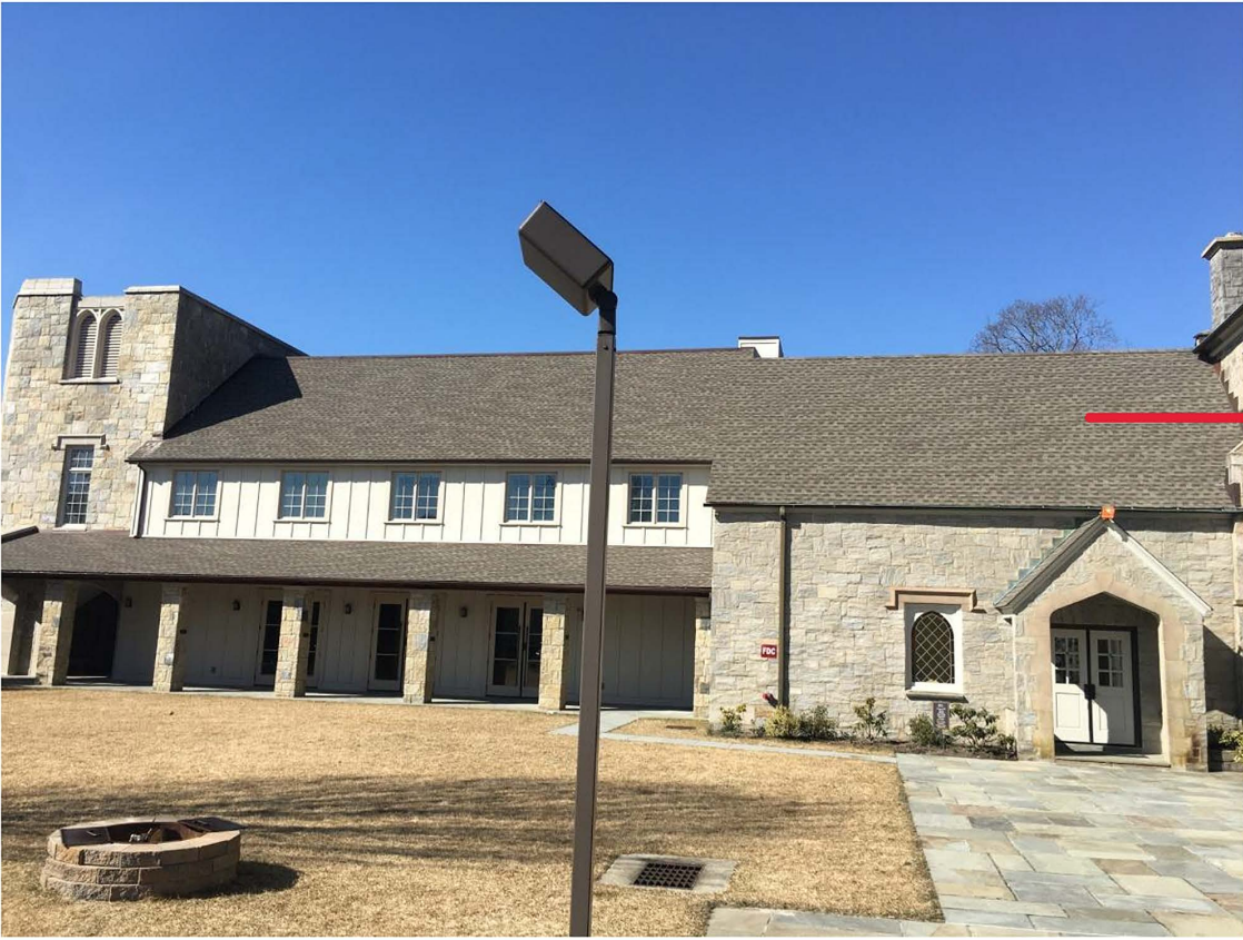
Weathered wood on C&HT existing roof
