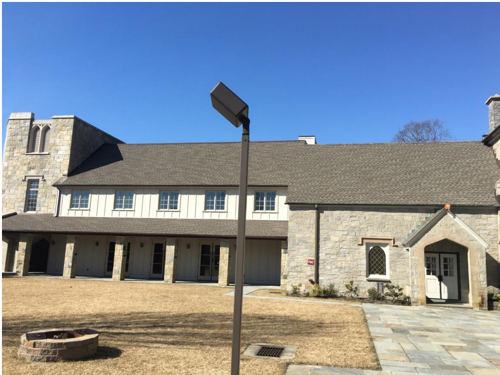
CHRIST & HOLY TRINITY CHURCH, Timberline "Weathered Wood" asphalt shingles on Branson Hall and stone connector to original building is the selection for the new roof on the stone church building.
