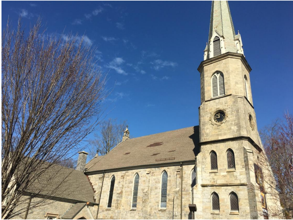
CHRIST & HOLY TRINITY CHURCH, View from Church Lane, showing the patched asphalt shingle roof to be replaced.
