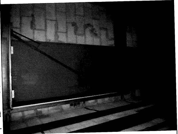
15 Hoistway Interior / Door Equipment
