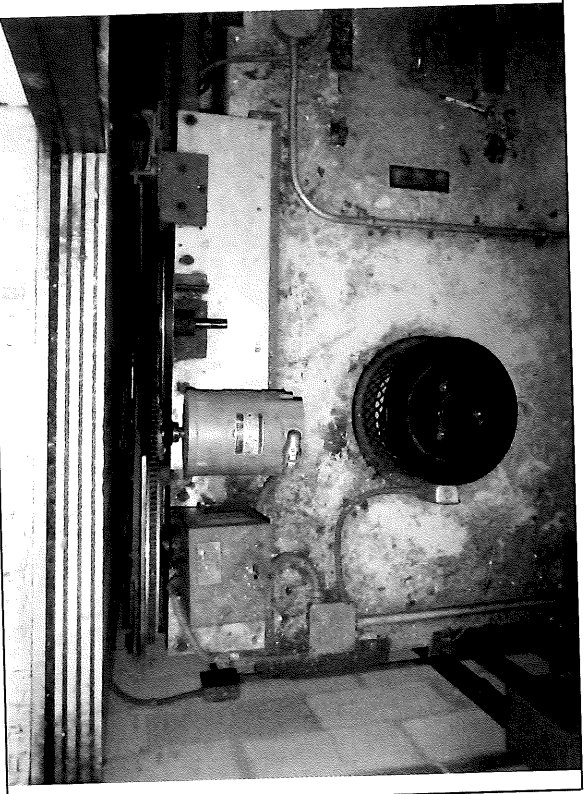
13 Top of Car – Door Operator and Cab Fan
