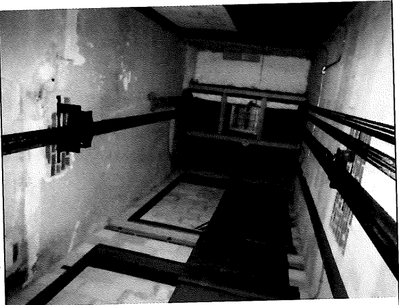
16 Elevator Hoist Way – Top of Hoistway Vent and Guide Rails
